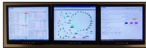
Ipswitch Atlanta NOC
